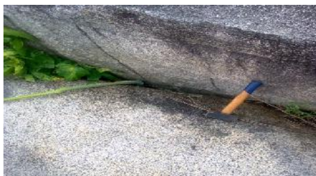
Fig. 5. An example of faults
