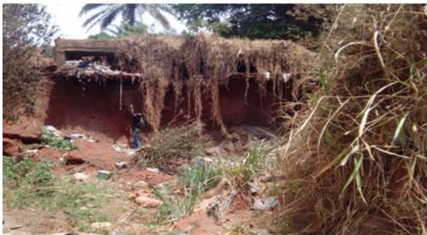
Plate E. Gully erosion at Onuiyi Road Culvert in 2016 (Note the author, whose height is almost half way the gully depth at 1.9 m)
