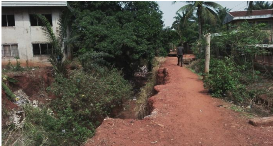
Plate H. Gully cut at Ibeziako Street with the street reduced to a footpath and house endangered by the gully in 2016
