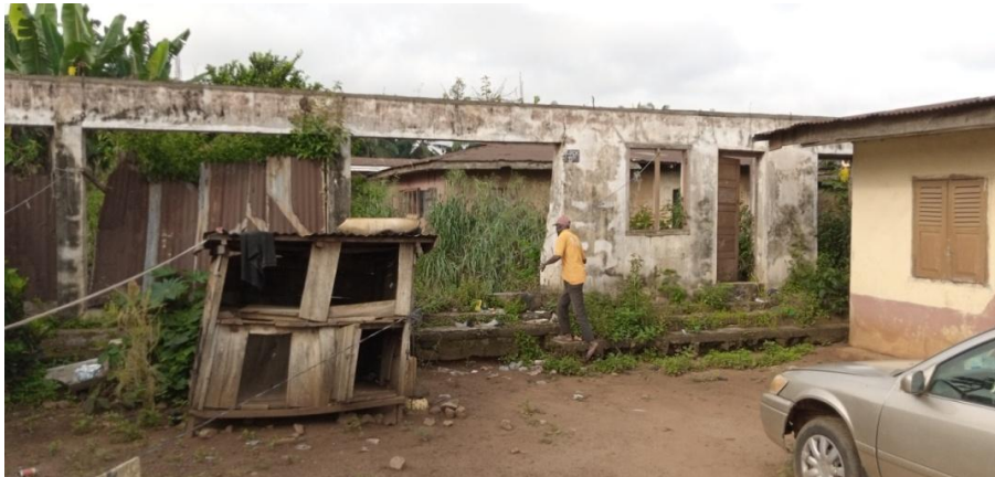
Plate L. The same property completely destroyed by the gully in 2020 Source: Authors Fieldwork, (2016 and 2020)
