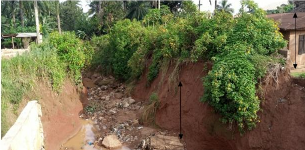
Plate F. The same gully erosion at Onuiyi Road Culvert in 2020 (Note the house around the gully site, with the height of the house about half of the gully depth at 3.84 m)
