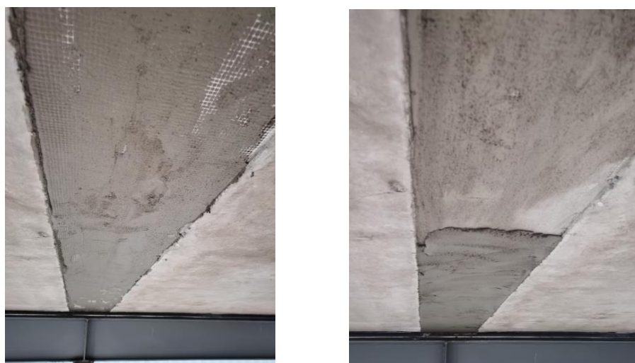
(g) Placing the alkali-resistant mesh fabric (h) Smoothing the bottom surface with mortar
