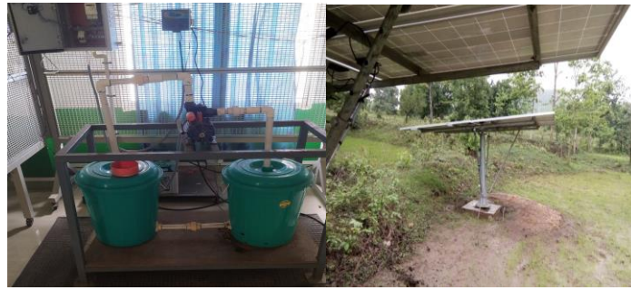
Fig. 9. Solar water pumps (1 HP and 2 HP Capacities)
