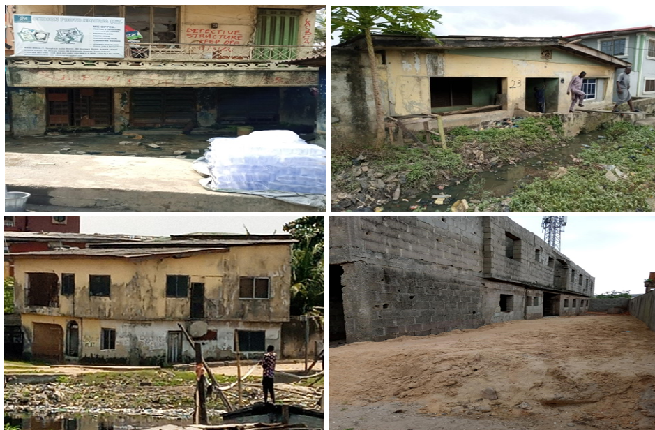
Fig. 1. Distressed buildings in the study area showing settlements and cracks on the buildings
